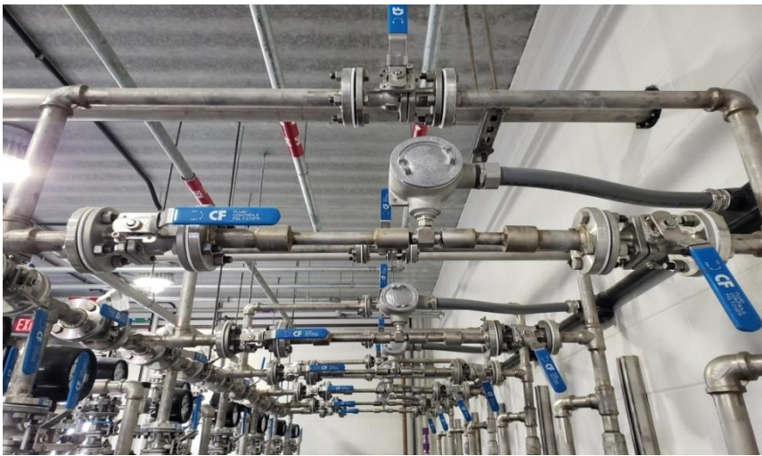
Methanol Injection Manifold
